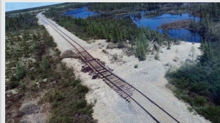
The destruction of the railway, due to which there was, in fact, the transport blockade of Churchill.
