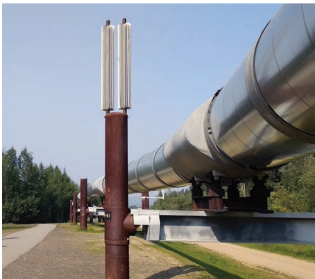
Figure 8.2. Thermosyphons alongside the Trans-Alaskan pipeline draw heat out of the ground and help keep permafrost temperatures low enough to support the above-ground structure. Alaska pipeline (2019). Photo: Nadezhda Zamyatina
