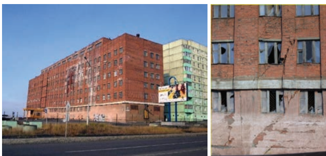
Figure 8.4. Building damaged by permafrost degradation, Norilsk, Russia. (Photo from 2013, now the building is dismantled). Photo: Nadezhda Zamyatina
