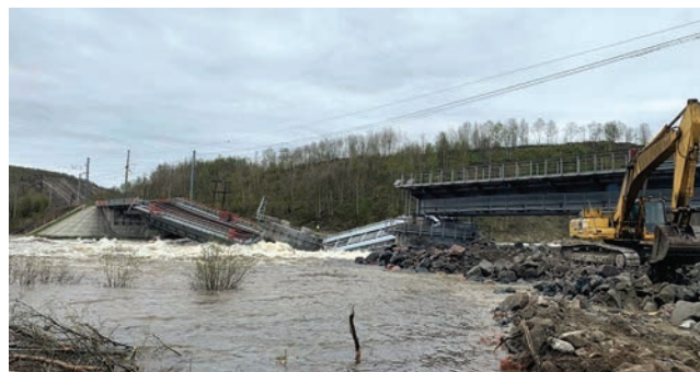
Damaged bridge near Murmansk interrupted railway communication with the regional capital
